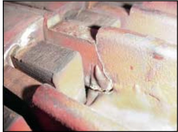
Fractures at the bar-to-end ring connection are common in fabricated rotors.
