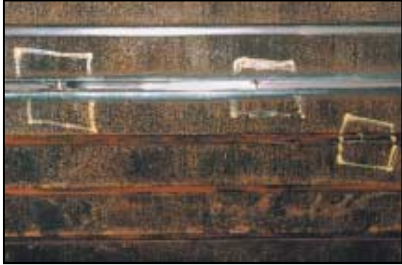
A cracked rotor bar that could be detected by tap testing or dye penetrant testing.
